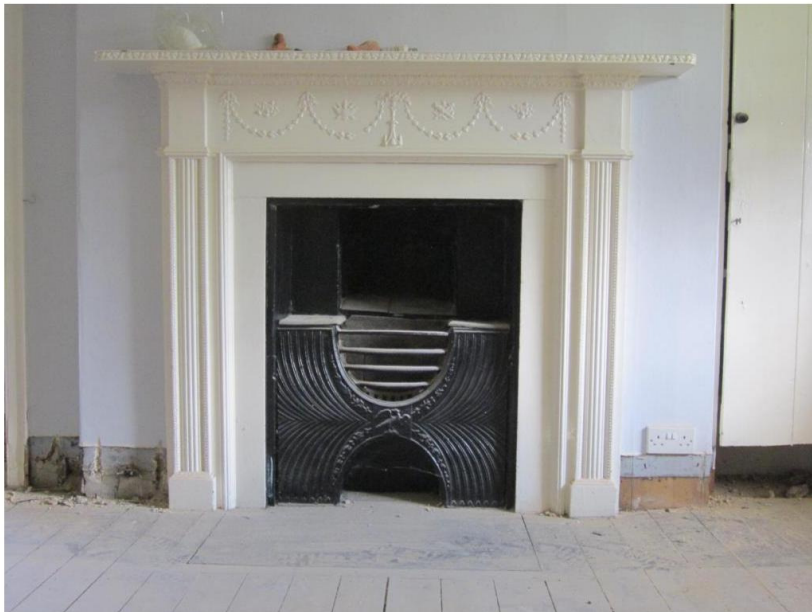
Fig 7 Building 1 Forest pattern hobgrate
